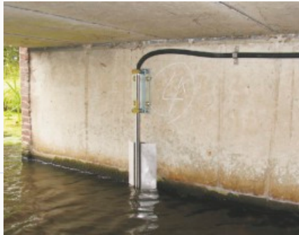
Installed rod sensor with accessories
