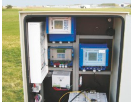
Clearly installed in a switching cabinet
