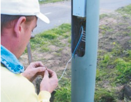
NivuChannel power supply using the street lighting
