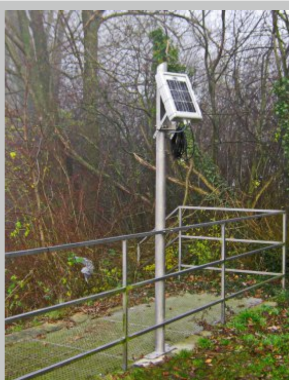
NivuLog SunFlow installé
